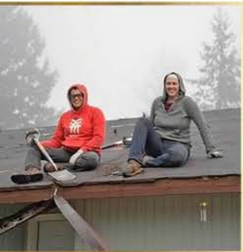
Kate and a local friend stripping off the roof of our house.
